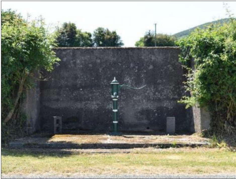
Figure 148 Water pump at Bunnagurragh
