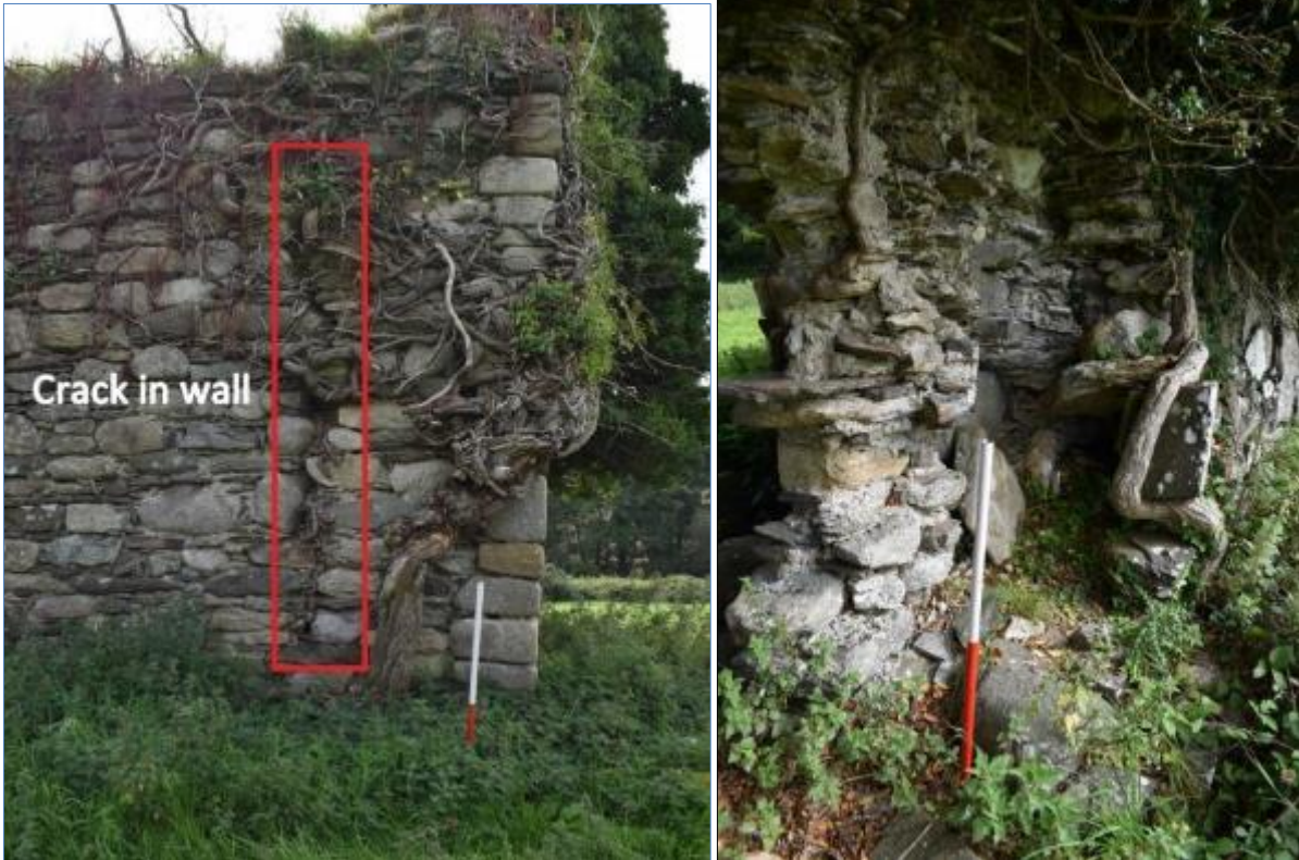
Figure 46 Substantial crack in northern wall and masonry void in southern wall
