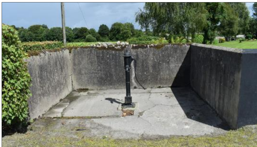
Figure 1046 Water pump, Crowsgrove
